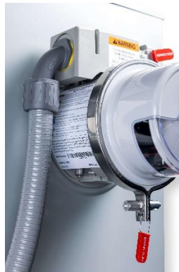
Figure 3: Meter socket providing power to a load (such as an EV charger)
