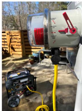
Figure 4: Transfer switch connected to a generator
